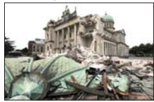
Rubble is seen in front of the severely damaged Cathedral of the Blessed Sacrament in Christchurch, New Zealand.
